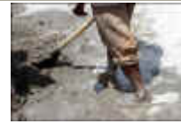
Mixing concrete in bare feet. It didn't occur to us that the villagers had no shoes that would be suitable for this kind of work.
