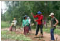
The villagers digging land to fill in either side of the bridge.
