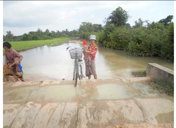
One of many damaged culverts.
